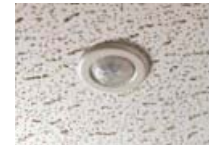
Ceiling Occupancy Sensor
